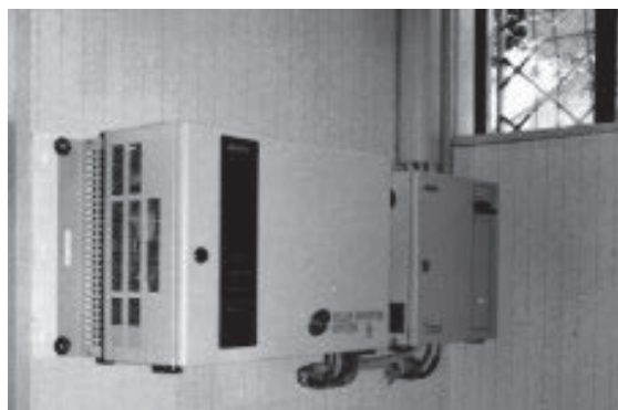
Fig. 6 Photo of the power conditioner.
