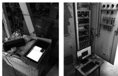
Fig.4 Measurement of Temperature and Pump operation.
