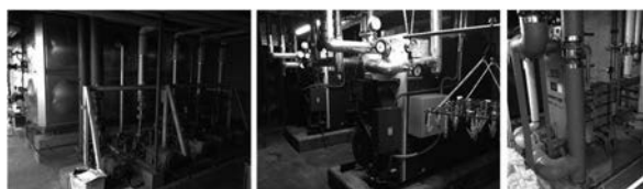
Fig.3 Thermal storage tanks, boilers, heat exchangers.
