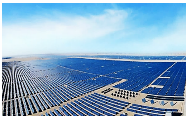
Fig.10 The world's largest solar power station in Qinghai province
