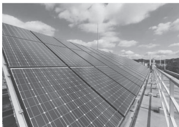
Fig. 4 Appearance of the photovoltaic generation system.
