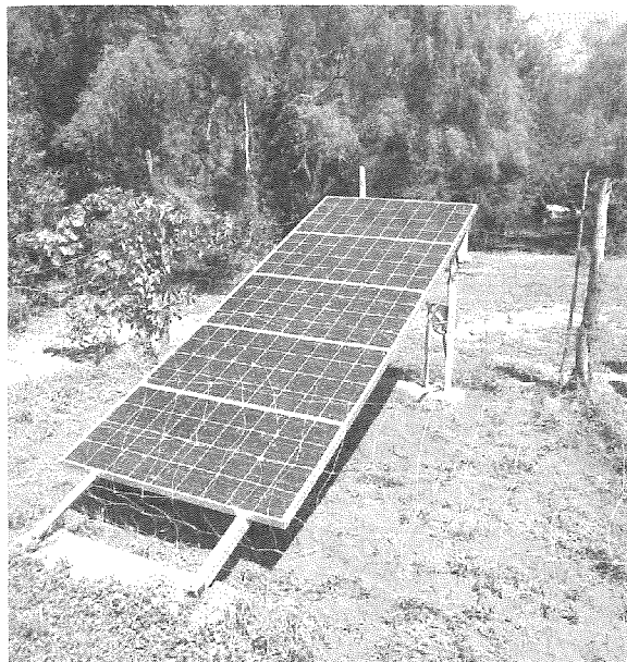
Fig.20 PV module installed in farm in Mexico
