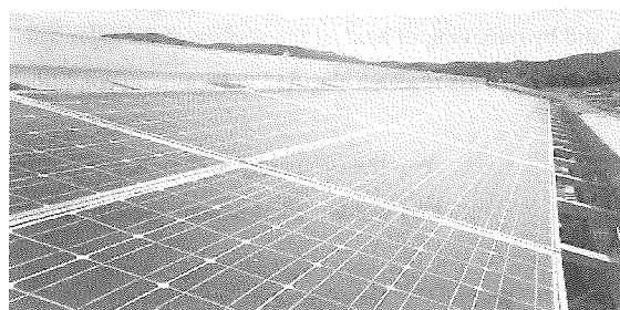
Fig.3 Solar panel with heat exchanger: C1
