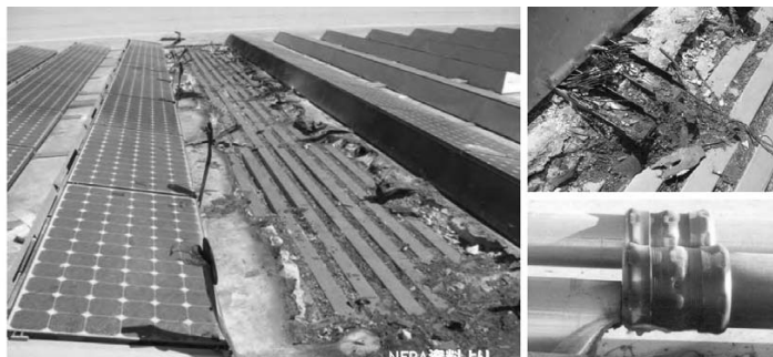
Figure 3 shows the second fault in a fire similar to the Bakersfield event. In this scenario, the short circuit current is forced through the small 10 American wire gauge (AWG) grounded string conductor, causing a conductor insulation fire. Figure 4 shows the second fault in a fire similar to the Mount Holly event, in which the array short circuit current is forced through the poor inadvertent grounding connection, causing an arcing fire.
