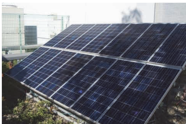
Fig.3 Appearance of PV system
